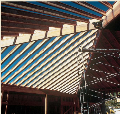
Long lengths turn dramatic spans and stunning designs into reality, as shown in this church roof under construction.
