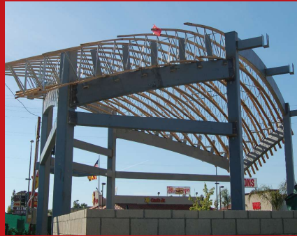
Open-web trusses allow for greater architectural flexibility, such as the curved roof of this quick-service restaurant in California.
